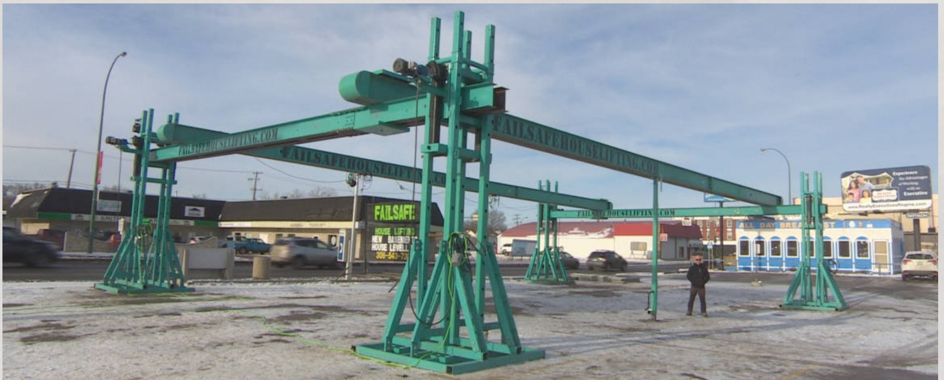
Wensel said his patented lift allows equipment such as skid steers to work underneath a house after it has been lifted. (Dean Gutheil/CBC)
